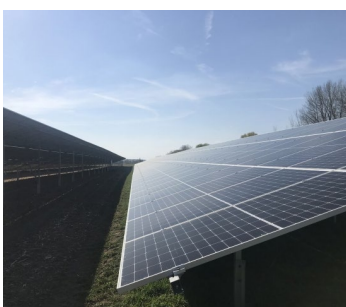
Photovoltaikanlage in Neuburg
