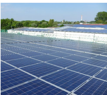
Photovoltaikanlage in Neuburg
